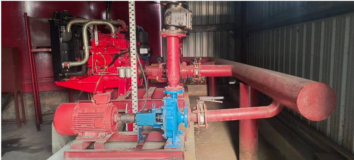
FIRE FIGHTING SYSTEMS
