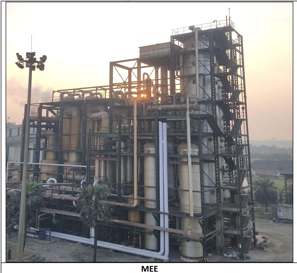
Photograph of the Centrifuge Decanters, MEE, Dryer, CPU, WWTP, RO Plant, DDGS godown, STP Plant
