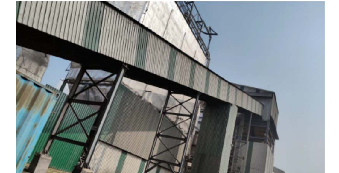
covered conveyer belt
